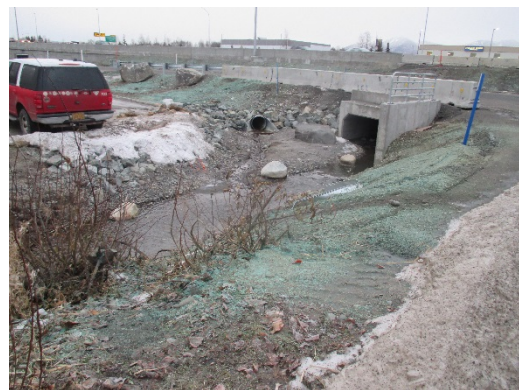
South Fork Little Campbell Creek box culvert outlet lacking down-slope sediment control measures/physical controls
