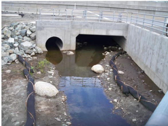
North Fork Little Campbell Creek box culvert with down-slope sediment control measures. (DEC Photo 26)
