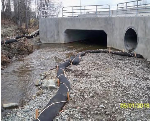
Compost sock installed by edge of creek near inlet of North Fork Little Campbell Creek. (DEC Photo 25)
