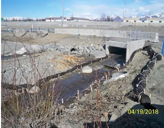
South Fork Little Campbell Creek box culvert outlet with down-slope sediment control measures installed prior to start of construction and spring thaw. (DEC Photo 12)
