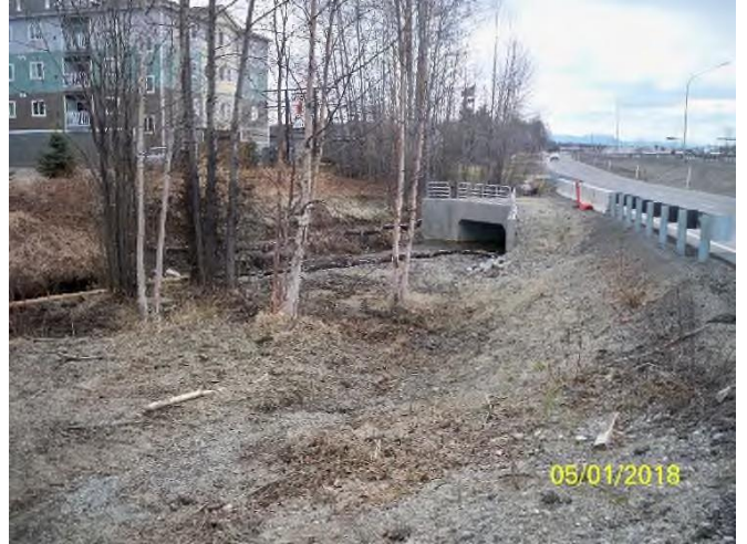
North Fork Little Campbell creek with down-slope sediment control measures installed prior to start of construction within proximity. (DEC Photo 23)
