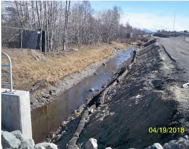
South Fork Little Campbell Creek reconstruction area with down-slope sediment control measures installed prior to start of construction and spring thaw. (DEC Photo 16)
